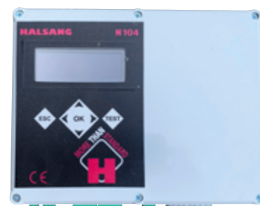
Electrical cabinet equipped with a Halsang H104 controller and frequency modulators
